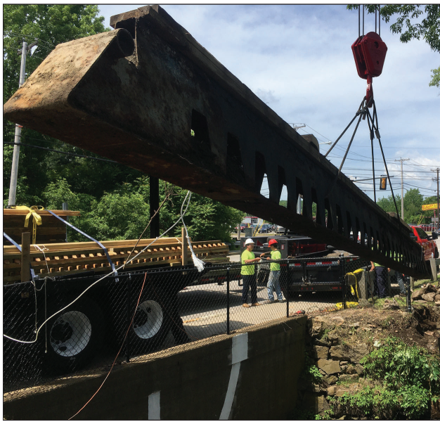
PUT INTO PLACE: Workers from JR Vinagro Corp., a Johnston construction company, used a crane to lower a prefabricated footbridge in place along Johnston War Memorial Park's walking path. The bridge work may be completed as early as Friday. (Photo courtesy Mayor Joseph M. Polisena)
