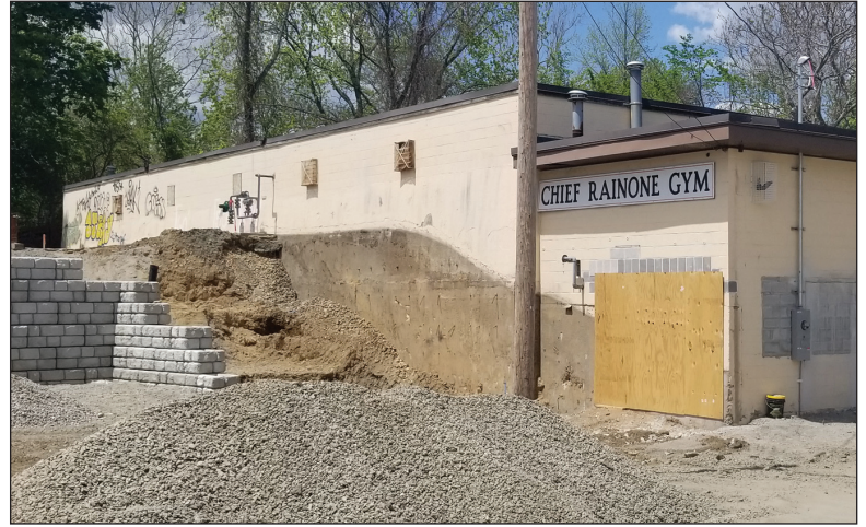
HARDWOOD: The Chief Rainone Gym, a 71-year-old facility at 45 Mill St., is undergoing a full renovation, inside and out. (Sun Rise photo by Rory Schuler)
